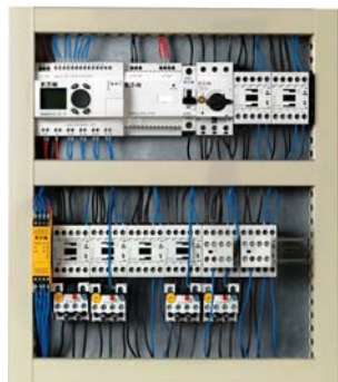
Panel with four traditional starters installed: FVNR, FVR, FVNR with E-stop and FVR with E-stop
